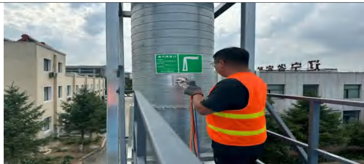
一车间排气筒 2DA007
