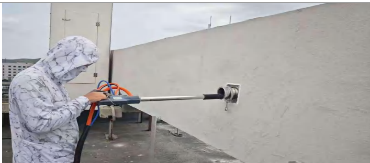
GLP 实验楼排气筒 2DA003
